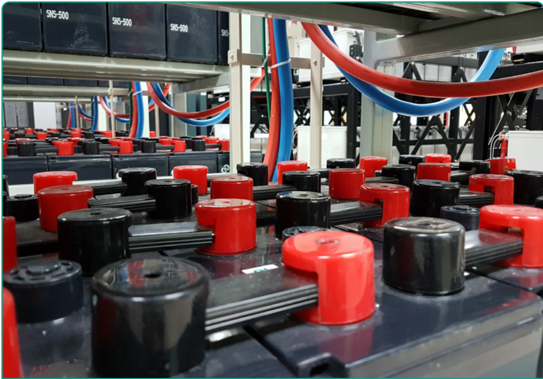
UNINTERRUPTED POWER SUPPLY
